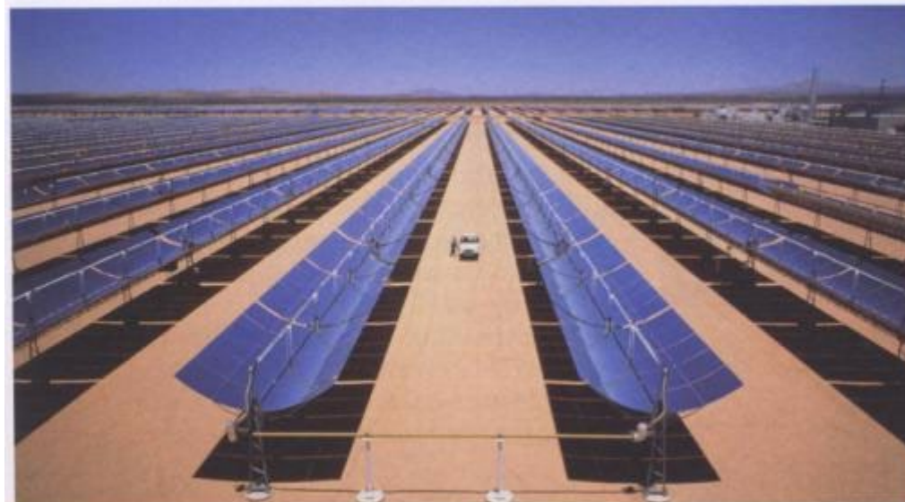
Figure 2.44 SEGS solar collector field at Kramer Junction in southern California
