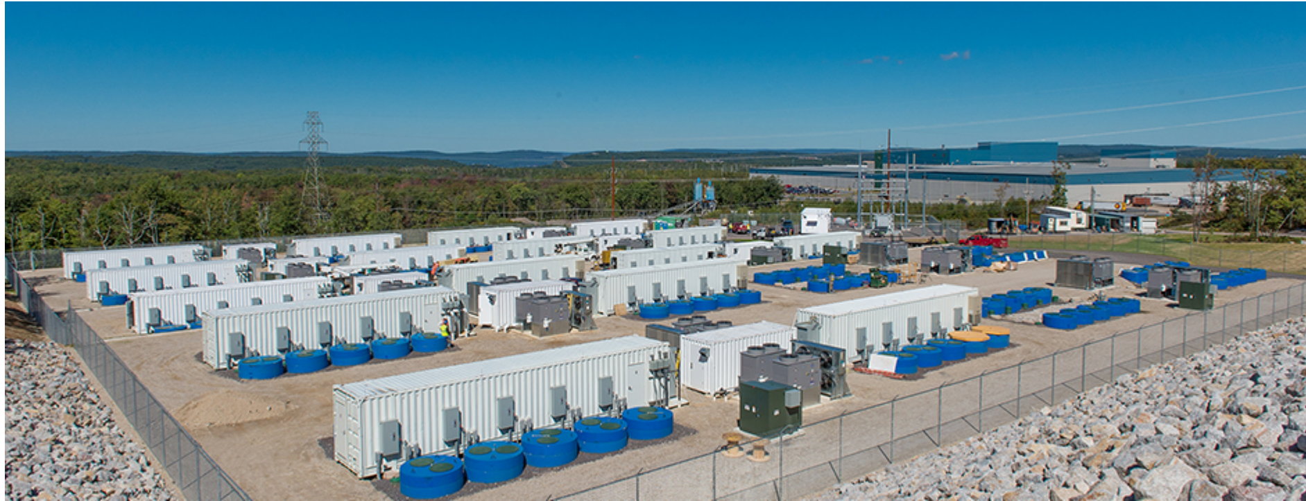
Hazle Township, Pennsylvania powerplant. Beacon Power©
