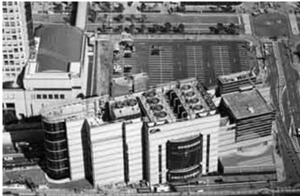
Figure 8.19 CTES system located on the roof of the technical building in Minato Mirai 21 ( Courtesy of Cristopia Energy Systems )
