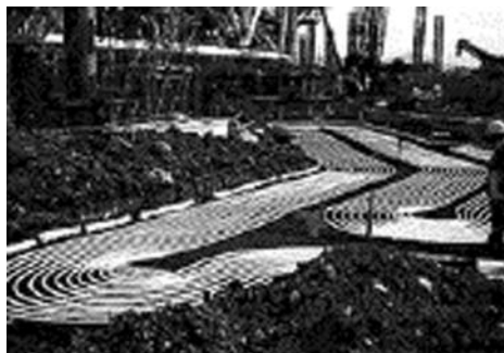
Figure 8.27 The network of water pipes with TES for heating and cooling buildings (JIN, 2000)
