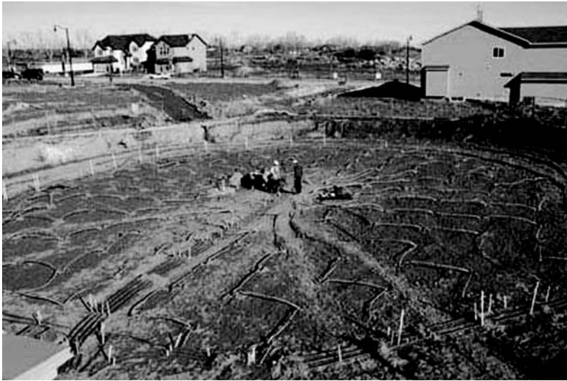
Figure 8.35 Construction photograph of the DLSC borehole thermal energy storage showing piping joining the boreholes in a radial configuration (Courtesy of DLSC). Source: “The Drake Landing Solar Community Project – Early Results.” B. Sibbitt, T. Onno, D. McClenahan, J. Thorton, A. Brunger, J. Kokko, B. Wong, Natural Resources Canada, 2007. Reproduced with the permission of the Minister of Natural Resources Canada, 2010
