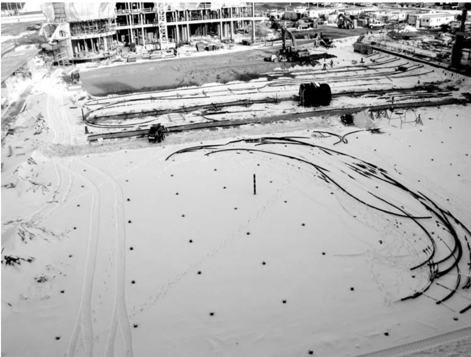
Figure 8.39 View of construction of the UOIT borehole thermal energy storage system, showing the grid of borehole headers and interconnecting piping
