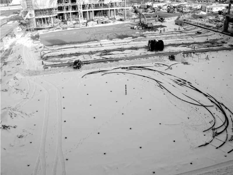
Figure 81. A site view during construction of the BTES at UOIT, showing the grids of boreholes and piping that interconnect them
