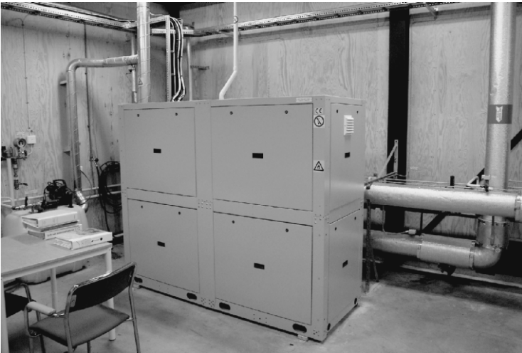
Figure 84. The heat pump inside the Energy Central
